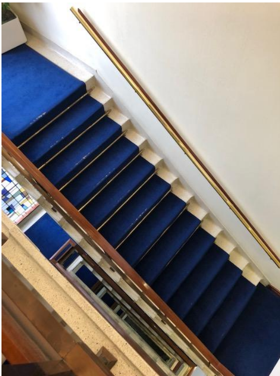
Fully intact terrazzo staircase of Building B that extends from fifth floor to basement
