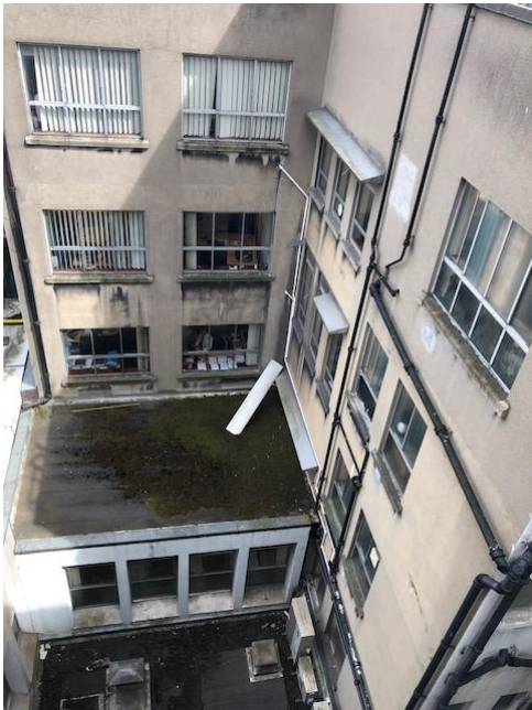
Rear of Building A onto Dawson Lane. Original Openings still intact along the rear elevation
