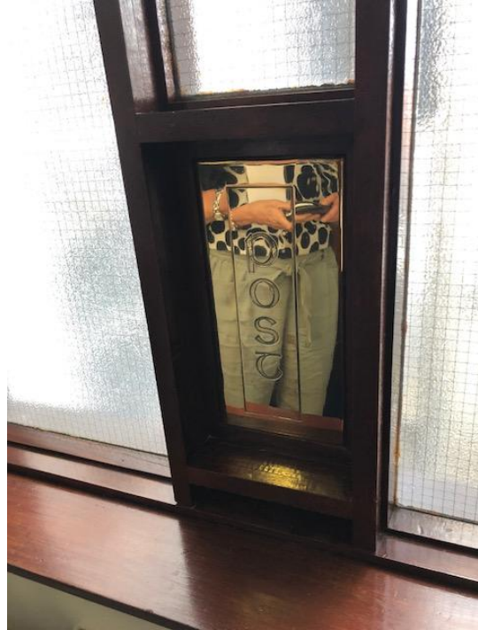
At each level, a letter box exists in the glazed link element between Buildings A and B
