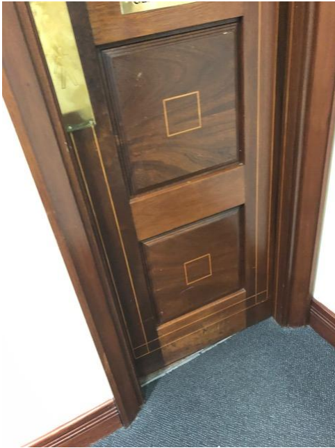
All joinery throughout Building A is identical. Doors with glazed panels have Georgian Fire glazing
